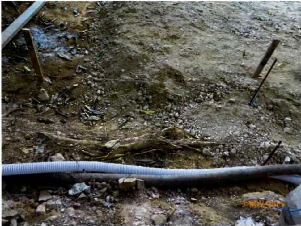
Fig 2. A large bare root has exposed on ground surface during inspection on 3 rd November 2015.
