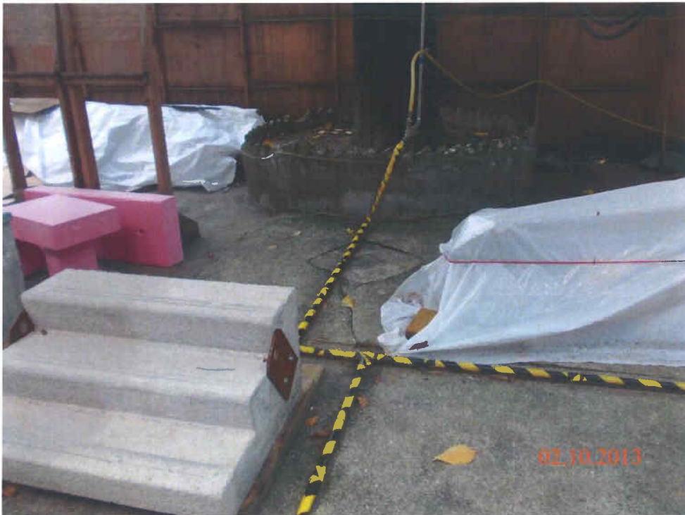
Fig. 3 Several heaps of construction materials are placed near the tree.
