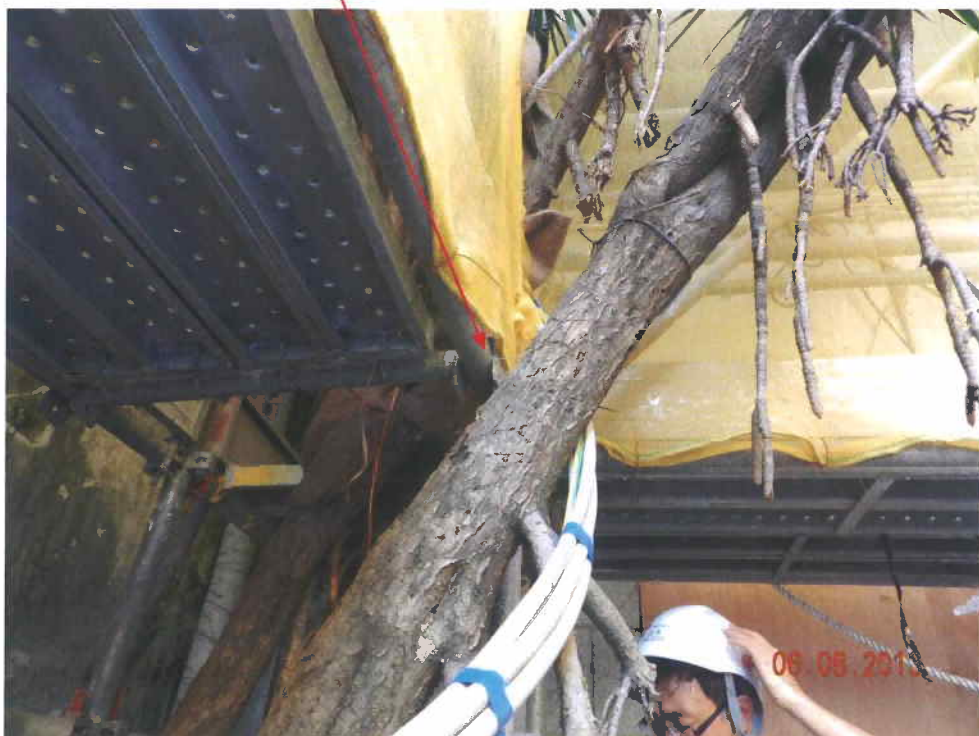
Fig. 5 The sharp edge of the scaffold still stabbed into the tree during inspection on 6 th August 2013.
