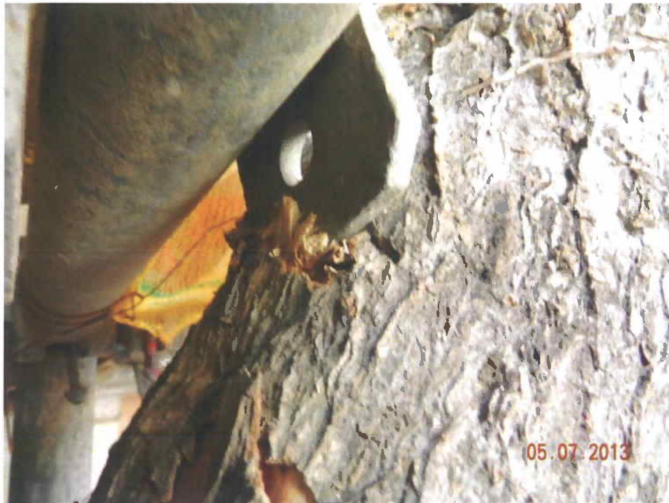
Fig. 4 The sharp edge of the scaffold was found to have stabbed into the tree during inspection on 5 th July 2013.
