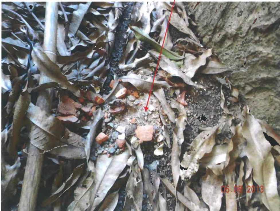
Fig. 3 The planter is full of fallen leaves and litter. Cleanliness of the planter is not acceptable.
