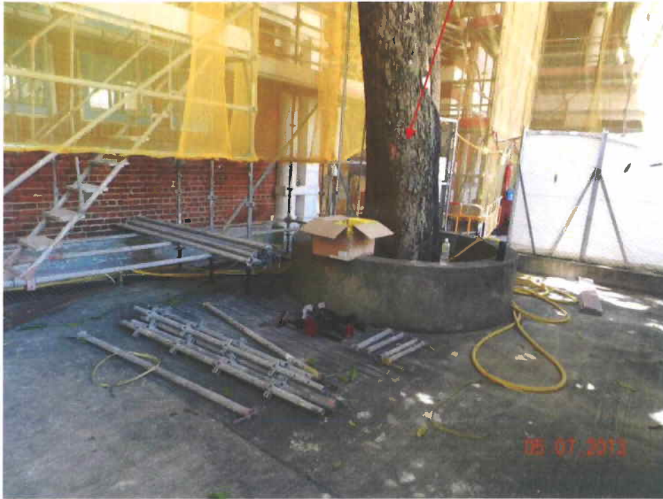
Fig. 4 Scaffolds had been set up inside the cordon zone. Many metal tubes were placed near Tree-5. Some wounds were found on the lower trunk during inspection on 5 th July 2013.
