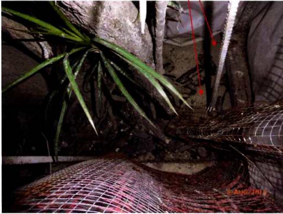
Fig. 2 Root collar is normal. Lots of wet cement appear at the planter.
