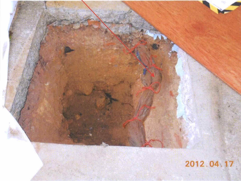
Fig. 6 One tree root , wrapped with hessian, appears at the trial pit.
