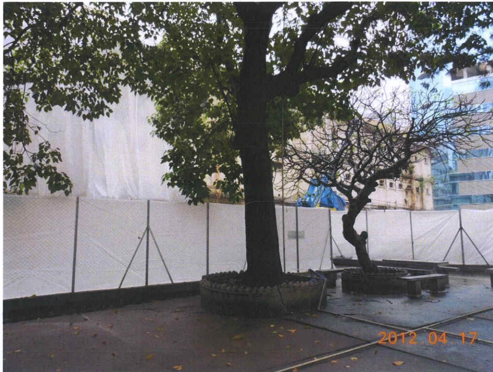
Fig. 4 The cordon zone keeps clean and tidy at the time of inspection.
