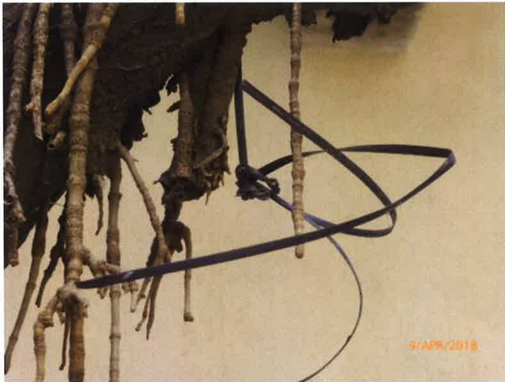
Fig. 8 A few construction debris remains on the tree.
