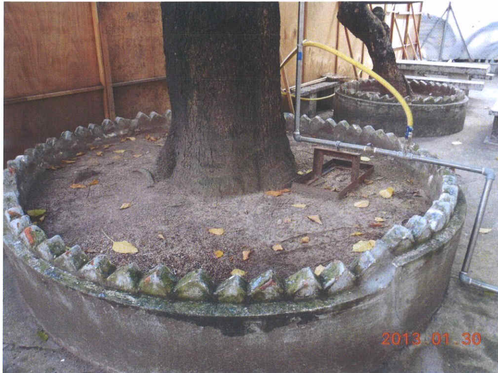
Fig 2. The planter is clean and tidy. No new cracks have been detected at the time of inspection.
