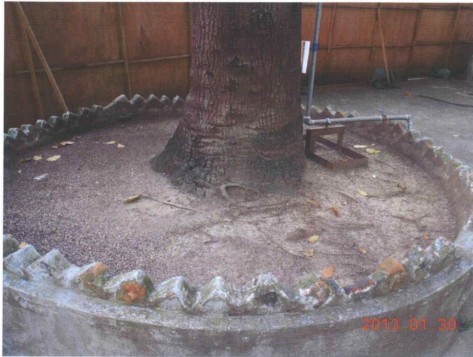
Fig 2. The planter is clean and tidy. No new cracks have been detected during inspection on 30.1.2013.
