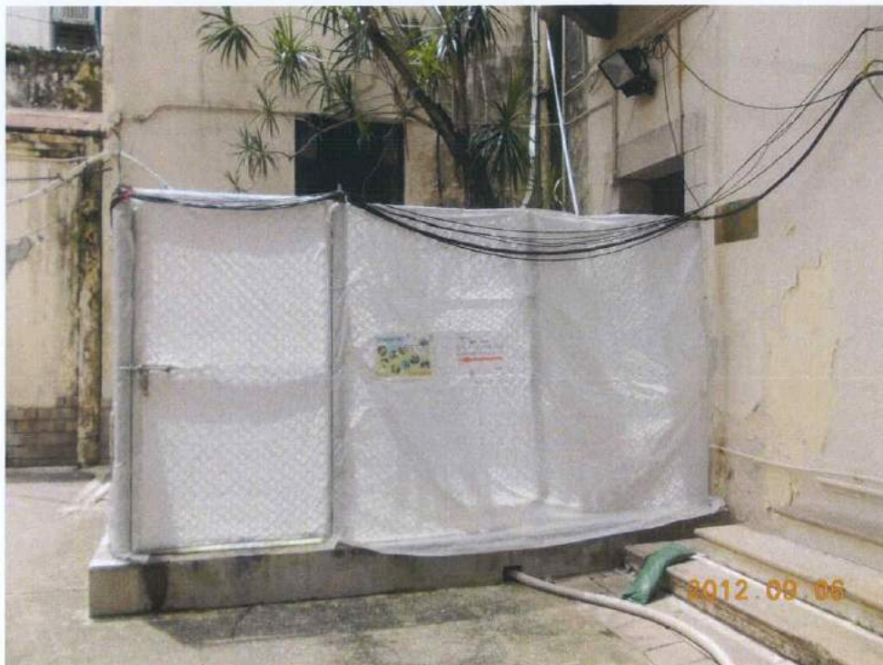
Fig. 5 The site outside the cordon zone is clean and tidy at the time of inspection.
