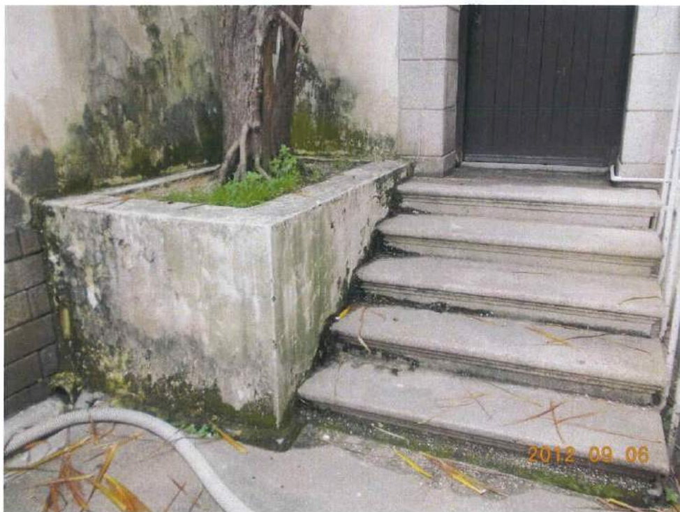
Fig. 3 Cleanliness of the site is acceptable and the wooden door is closed during inspection on 6 th September 2012.
