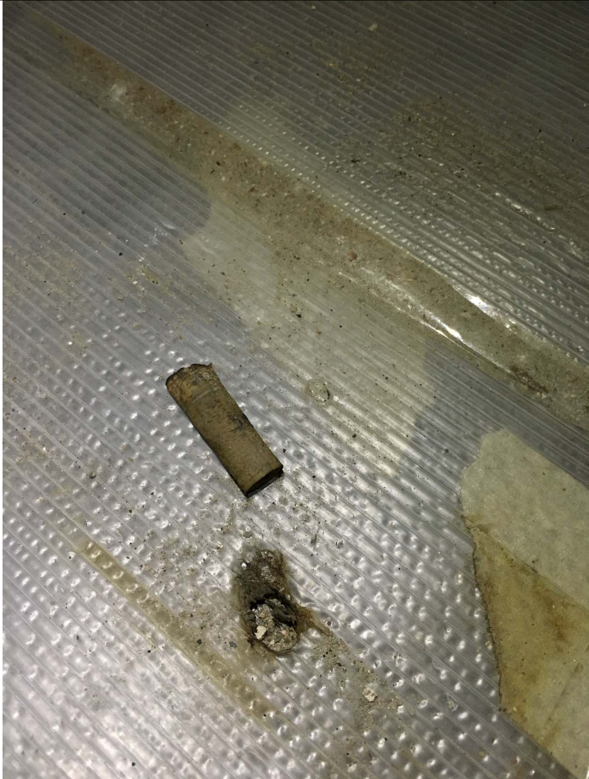
Above, photograph taken on 4 th November 2016, showing the damage by cigarette to the protection and the timber floorboards in room 03/F/22.
