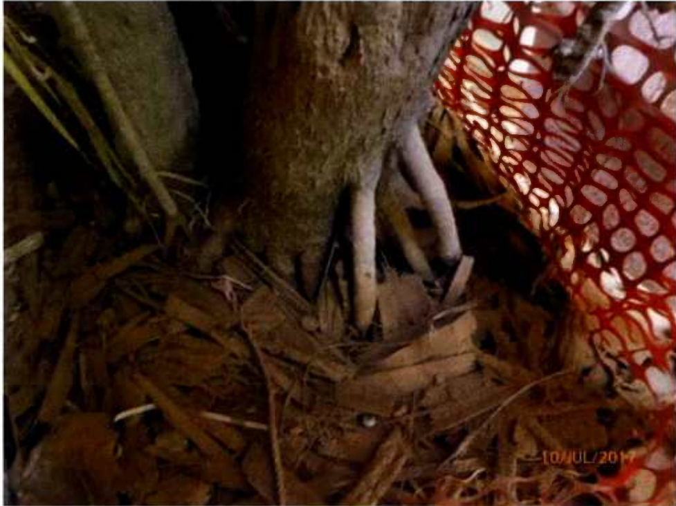
Fig. 2 Root collar is normal. The planter is covered with construction dust.
