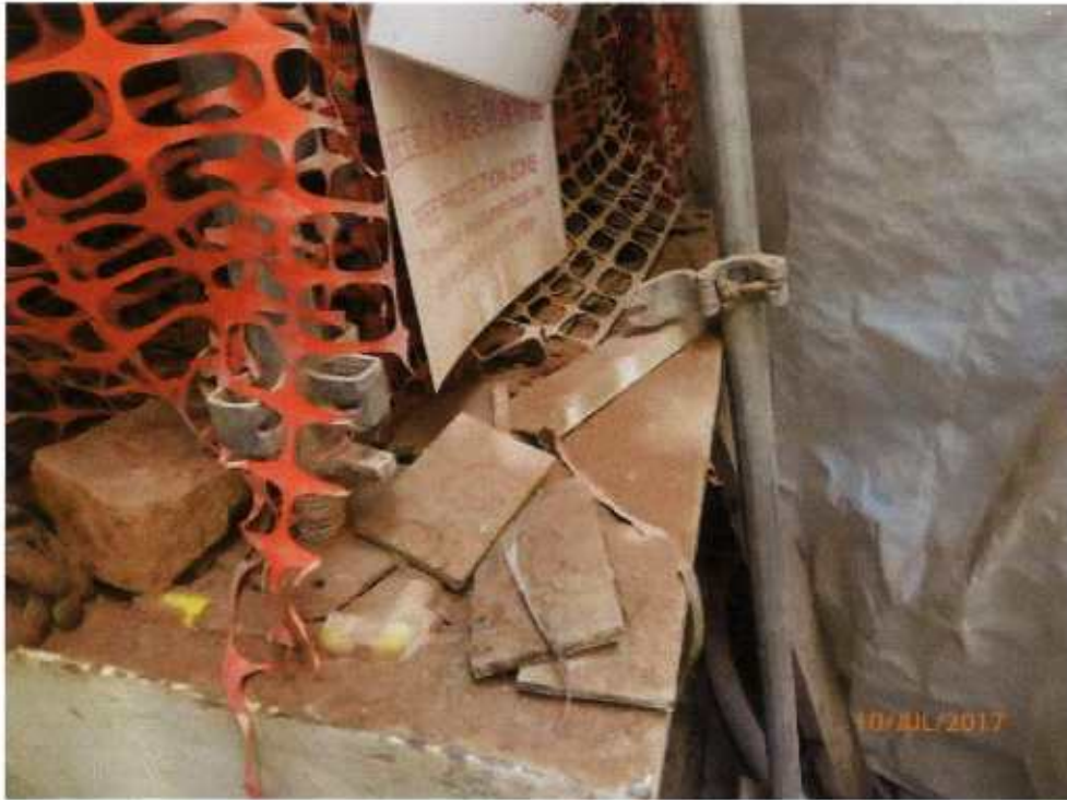
Fig. 10 Many construction materials are placed near the tree.
