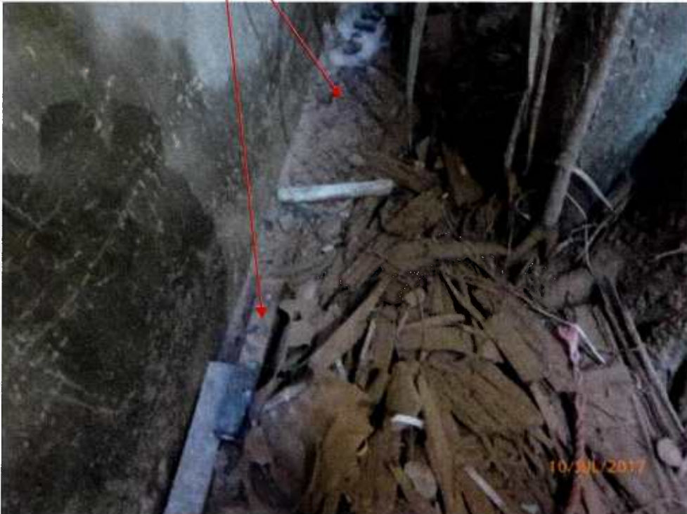
Fig. 3 Lots of construction debris scattered at the corner of the planter.
