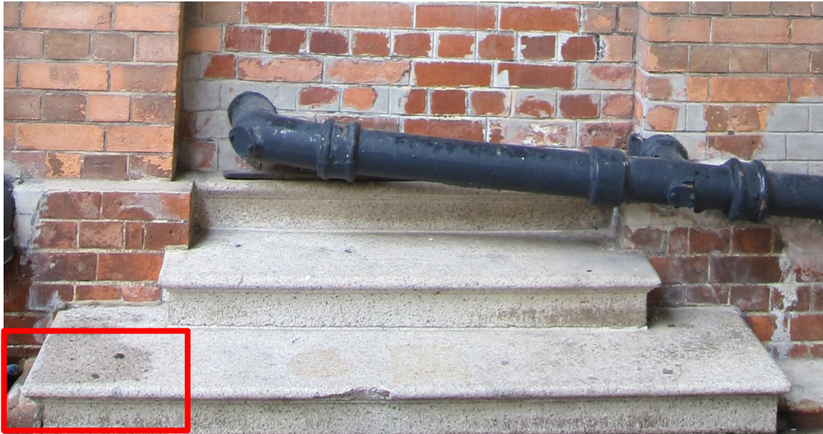
Above, photograph taken on 26 th April 2011, showing granite steps at 09/WG/04. The highlighted area was damaged during site works.
