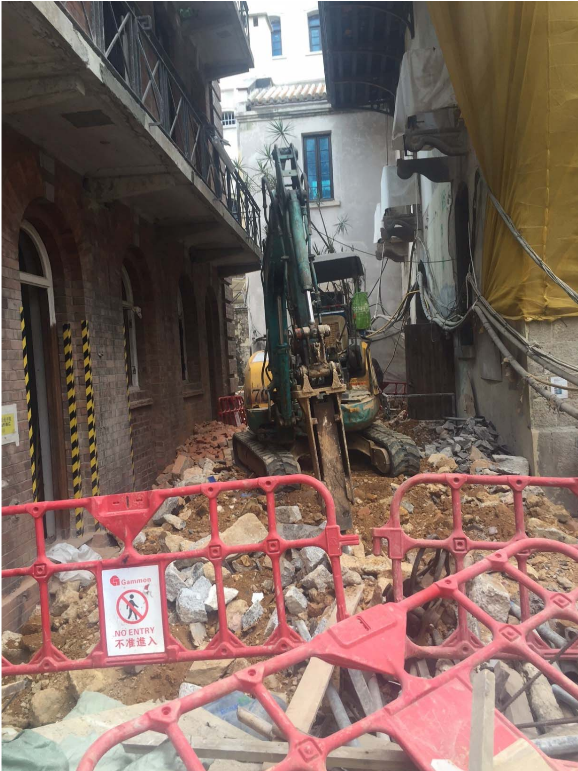
Above, photo taken on 5 th November 2015, showing site works on the Magistracy Terrace (West). No protection was provided to the granite steps nor the masonry walls.
