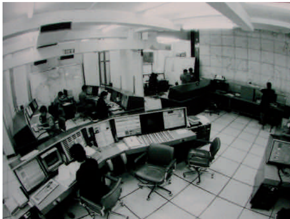
Radio Control Room
