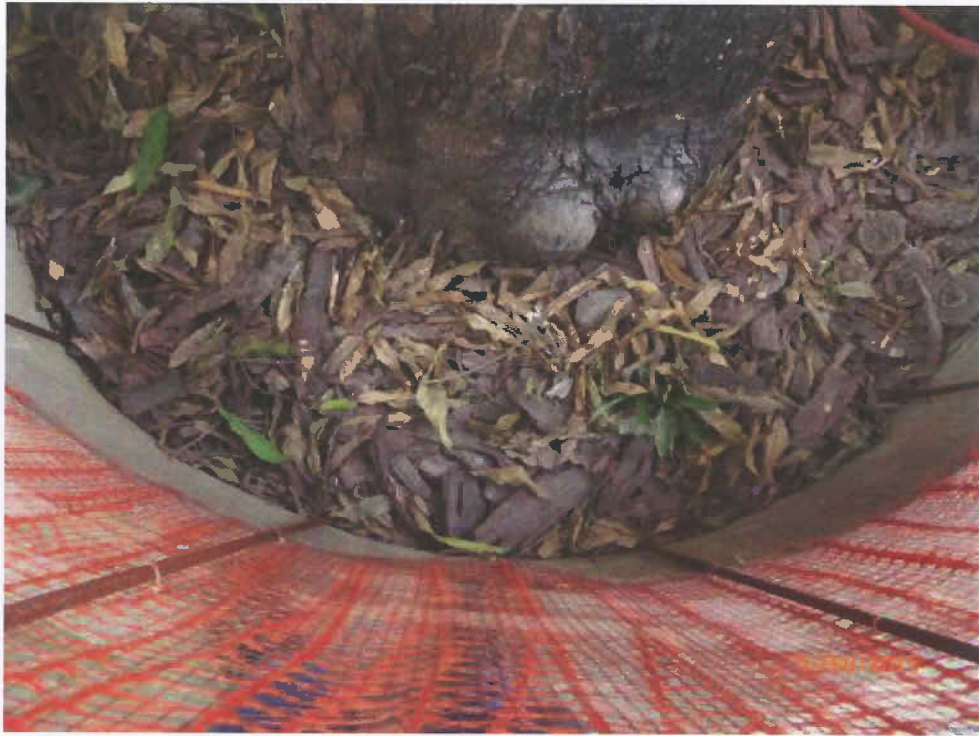
Fig. 2. Root collar of Tree-5 is normal. Reasonable mulch covers the planter.
