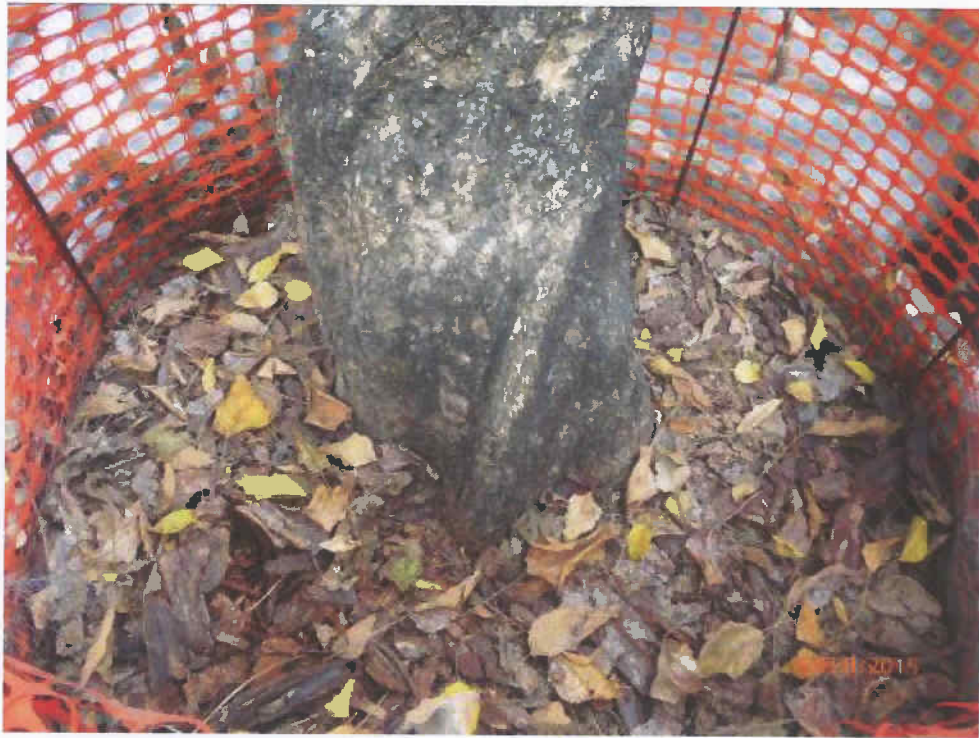
Fig 2. Root collar is normal. The planter is full of mulch and falling leaves.
