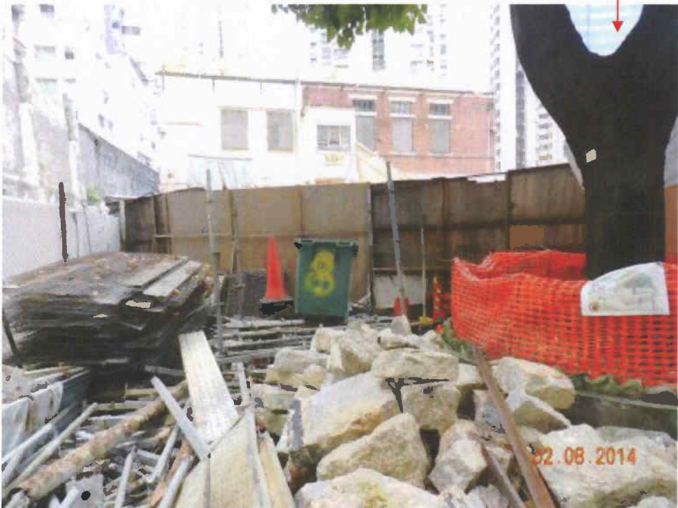
Fig. 7 Many construction items are placed near the planter. Tree-6
