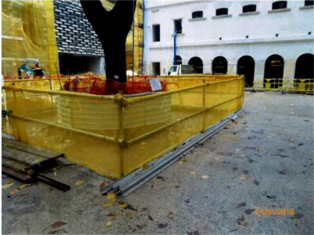
Fig. 12 A large cordon zone is newly set up near the tree.
