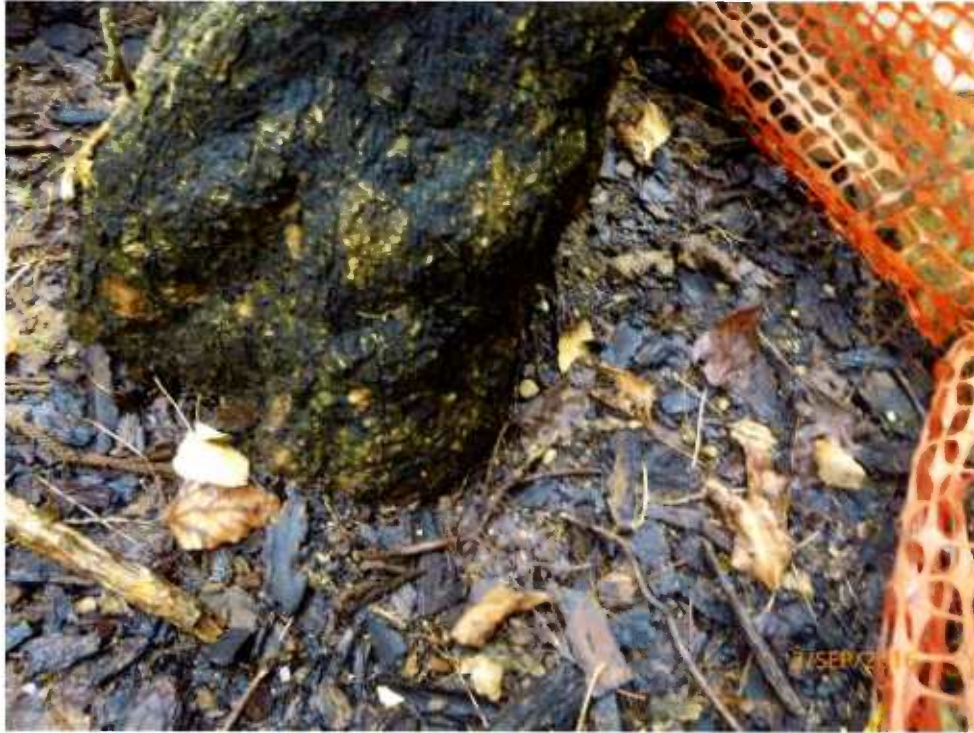
Fig 2. Root collar is normal. The planter is covered with mulch and leaves.
