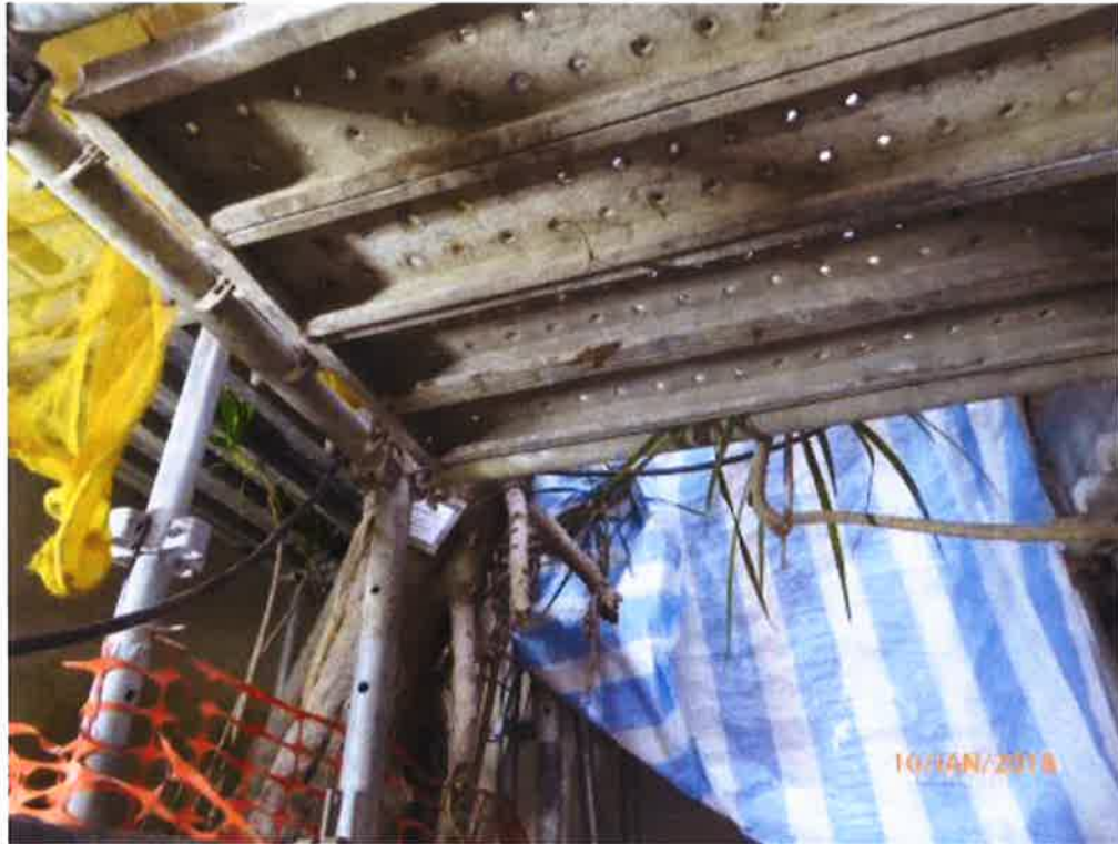
Fig. 10 Another large working platform also set up close to Tree-11 for renovation works.
