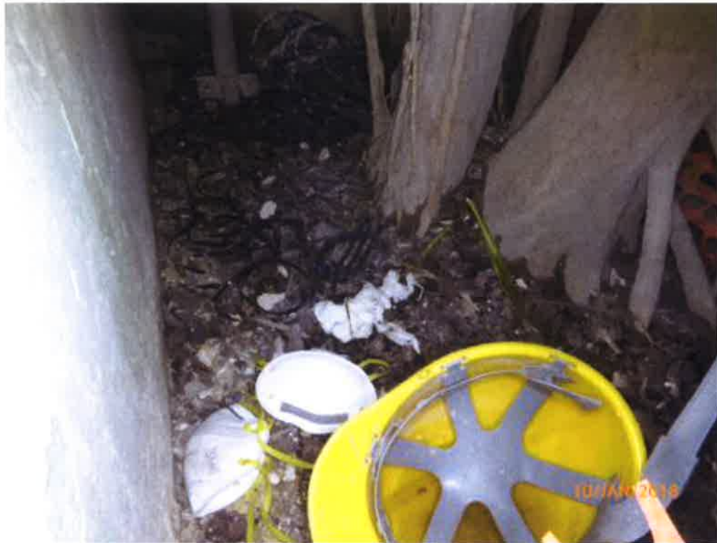
Fig. 2 Root collar is normal. A few construction debris remain at the planter.
