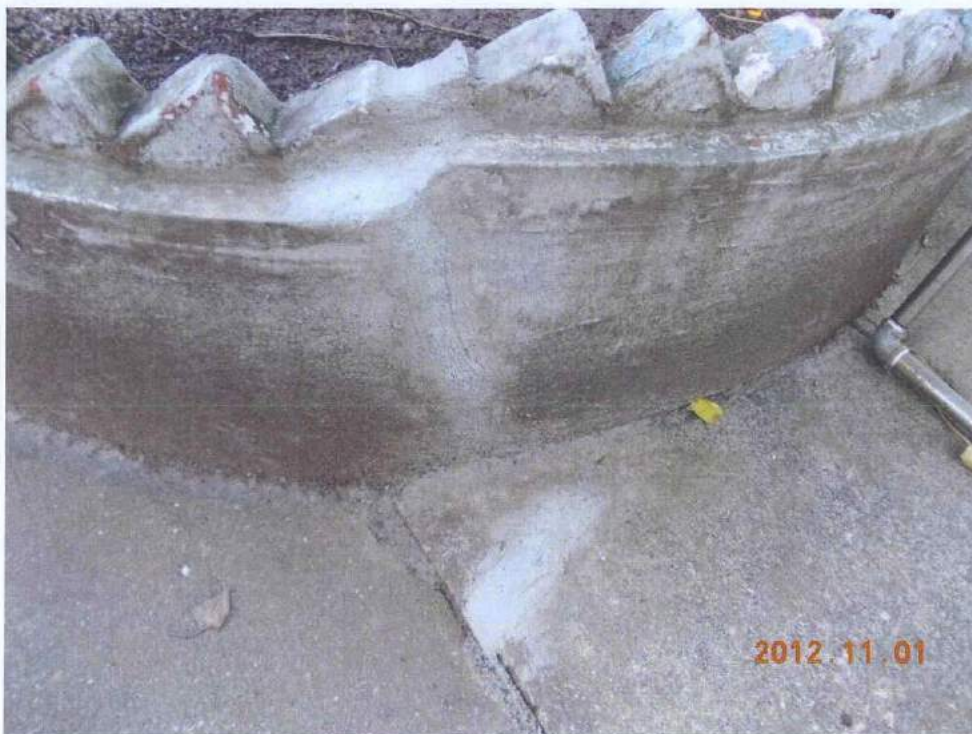
Fig. 3 The cracks in question are well-repaired. No more new cracks have been found at the time of inspection.
