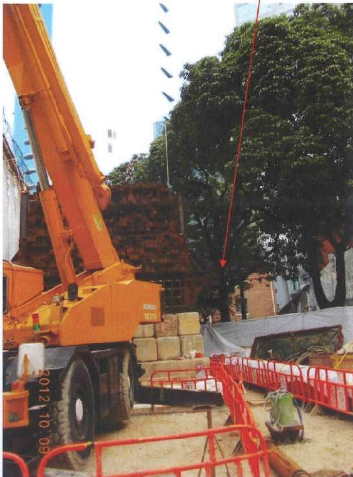
Fig. 6 Many bulky items were placed near Tree-7 on 9.10.2012.
