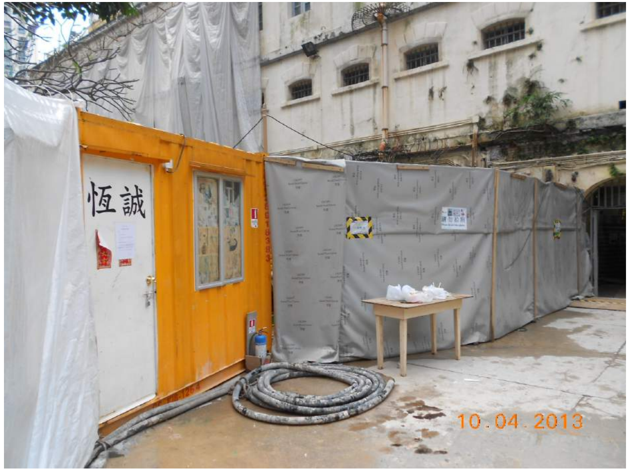
Figure 2 – Noise barrier for air compressors near Block 14
