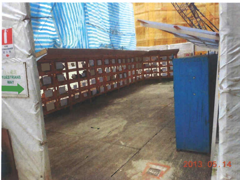
Fig. 5 Part of cordon zone has been altered to a worker store-room. Utmost attention to land pollution e.g. pouring of chemical liquid etc. should be paid at all times.
