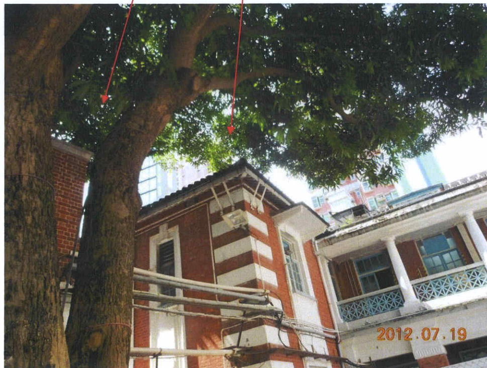
Fig. 5 Some lower branches and leaves are too close to the nearby buildings. Trimming of such branches/leaves is recommended..
