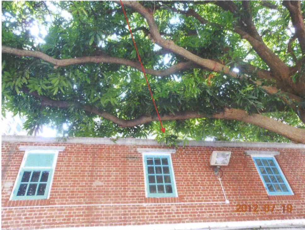
Fig. 4 Some lower branches and leaves are too close to the nearby buildings. Trimming of such branches/leaves is recommended.
