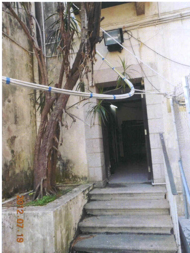
Fig. 3 The wooden door is found opened at the time of inspection.
