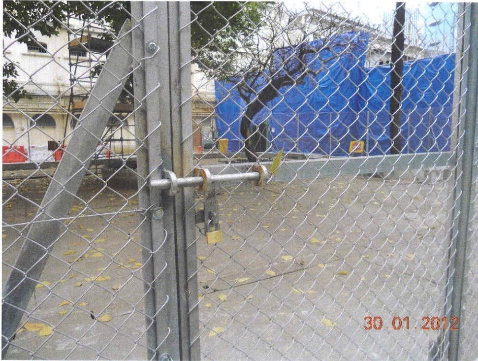
Fig. 6 Before leaving the site, the door has been properly locked and restricts admittance to the protection zone.
