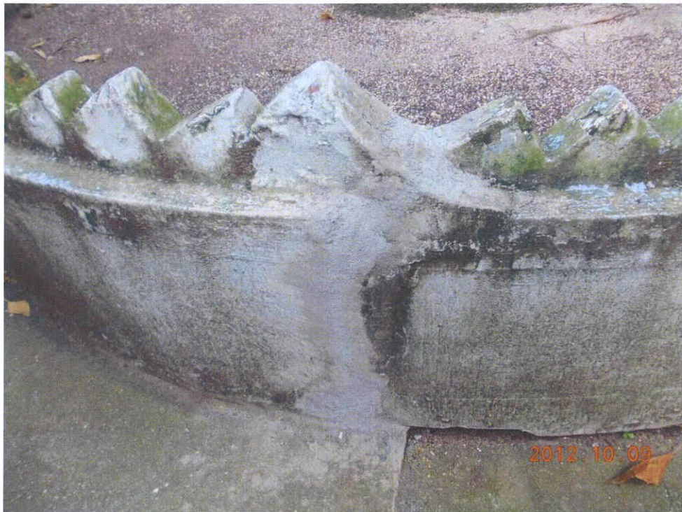
Fig. 3 Cracks in question are well-repaired. No more new cracks have been detected at the time of inspection.
