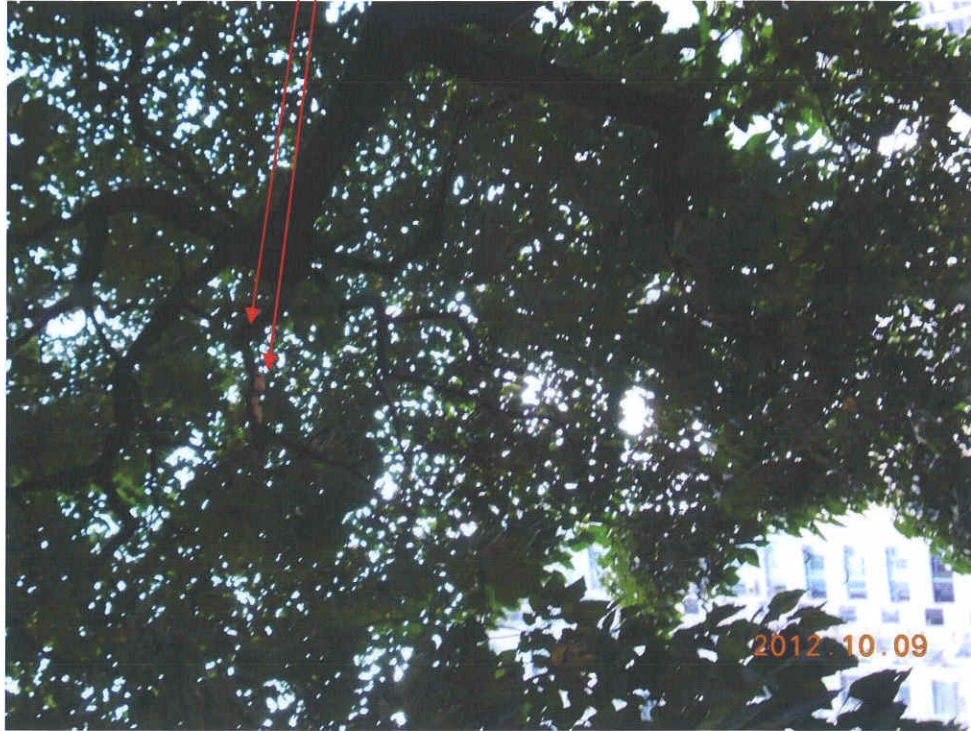
Fig. 6 Some decayed branches have been found on the tree top. Such decayed branches should be removed a.s.a.p.
